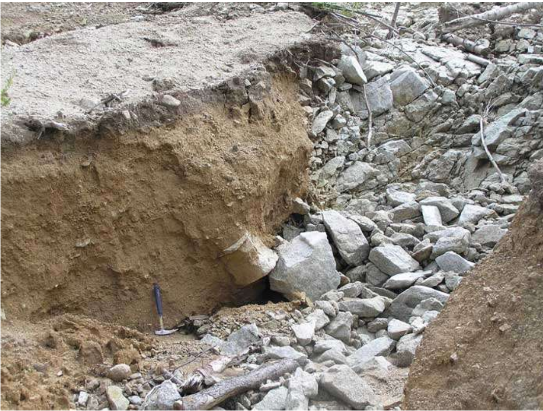
29. Ditches with depth of 1,8 – 2m, width up to 1,5 – 2m and length of 60 – 80m
