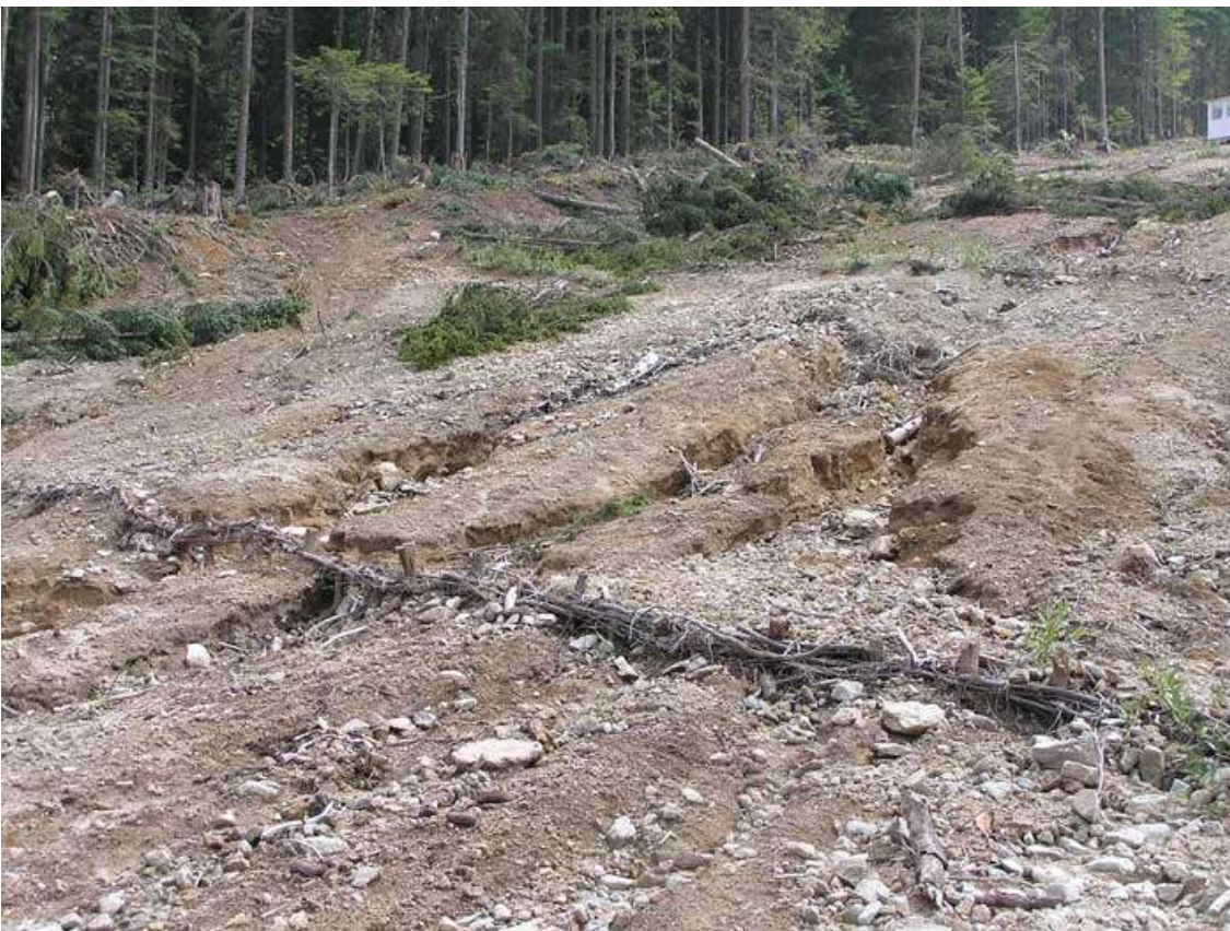
30. Ditches with depth of 1,8 – 2m, width up to 1,5 – 2m and length of 60 – 80m
