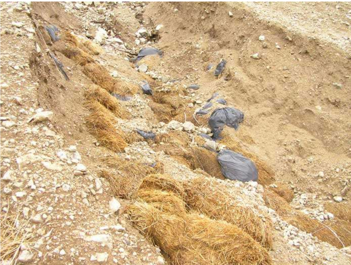
38. Insufficient anti-erosion measures
