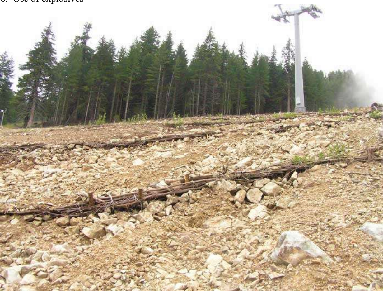
8. Insufficient anti-erosion measures
