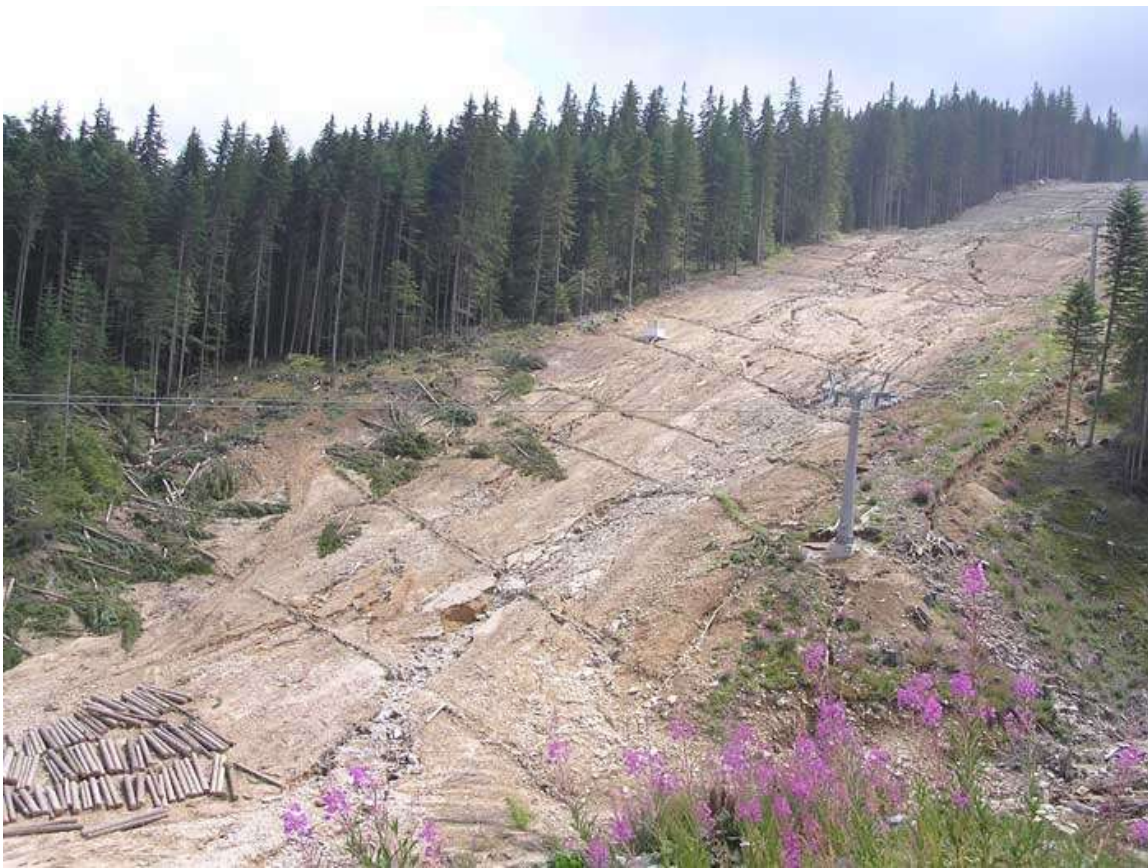
39. Insufficient anti-erosion measures
