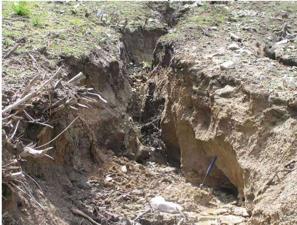
28. Ditches with depth of 1,8 – 2m, width up to 1,5 – 2m and length of 60 – 80m
