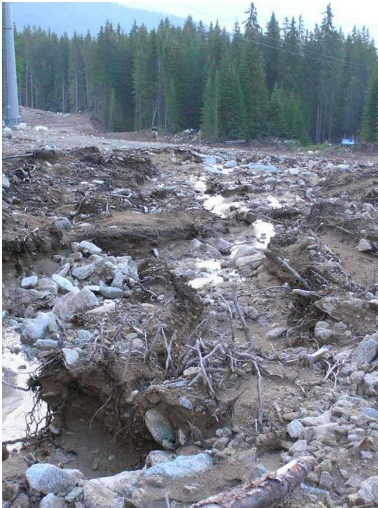
27. Ditches with depth of 0,7 – 1m, width up to 1,5m and length of 50 – 60m
