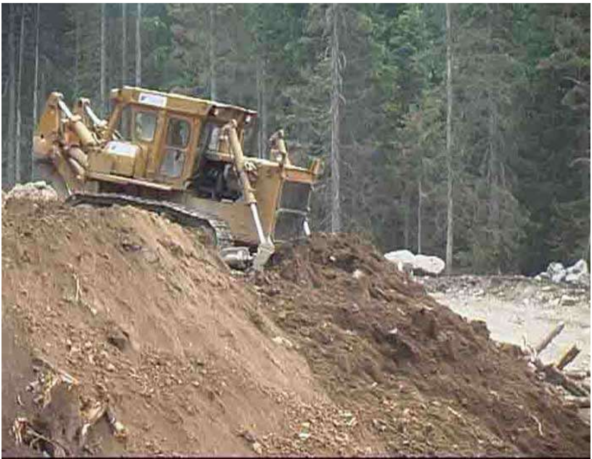
3. Illegal excavation work with heavy-chained machines
