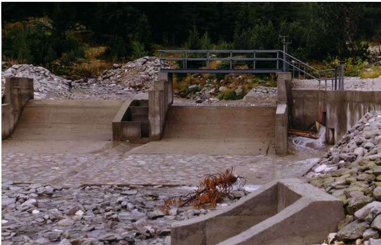
2. An illegal water catchment
